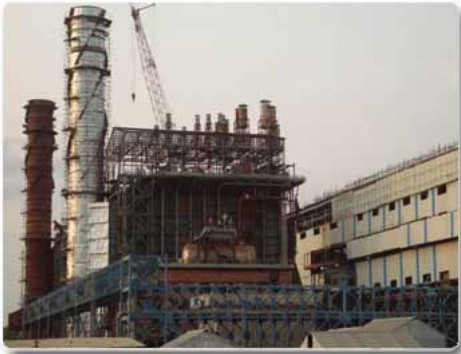
1090 MW Tripura Gas Based Power Project
